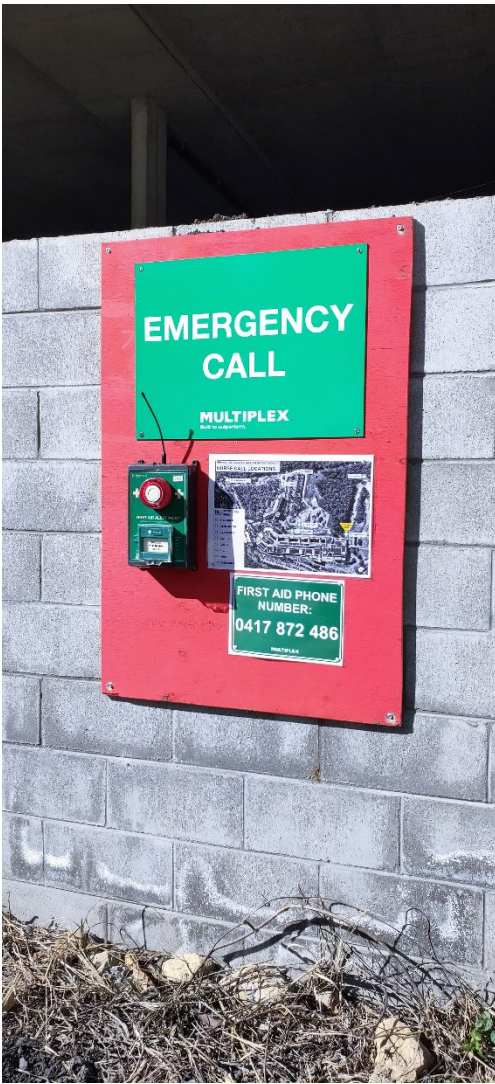
Photograph 3 – Emergency contact point
